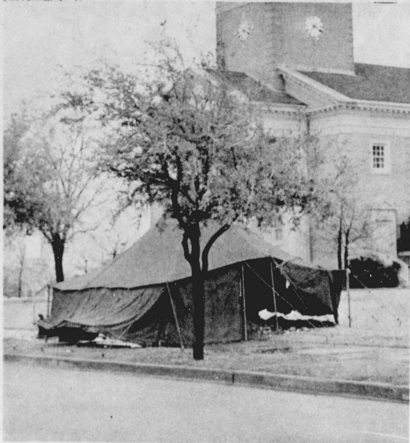
An ole' fashioned revival? Not really, it's just a weather shield for workers repairing defective underground power cables which recently put out lights in the library and other nearby buildings. Electrical power is being supplied by a temporary system. The tent is gone now; workers will finish repairs when the weather gets better, according to the Maintenance Department.
