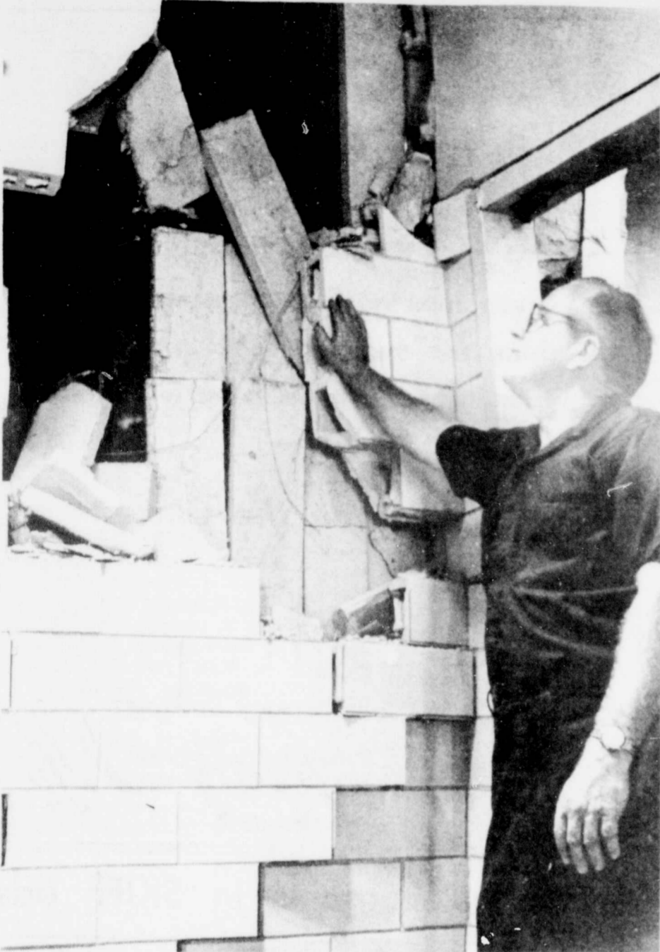
MAINTENANCE MAN EDDIE SCHMIDT EXAMINES DAMAGE It is estimated that repairs will cost $20,000
