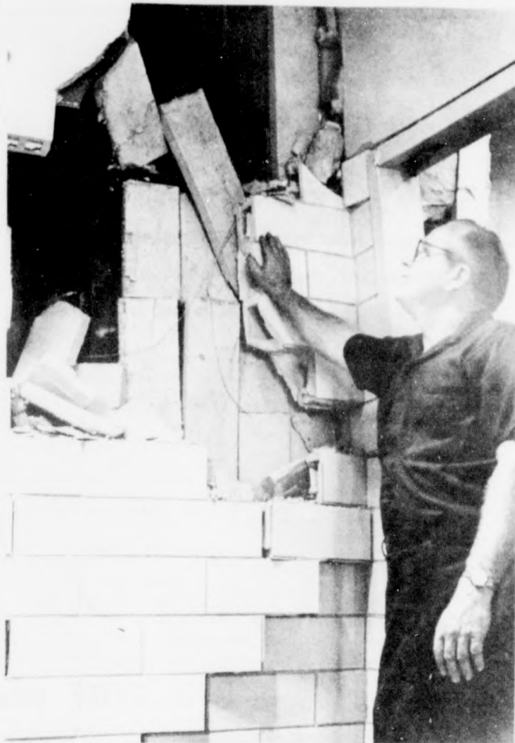
MAINTENANCE MAN EDDIE SCHMIDT EXAMINES DAMAGE It is estimated that repairs will cost $20,000
