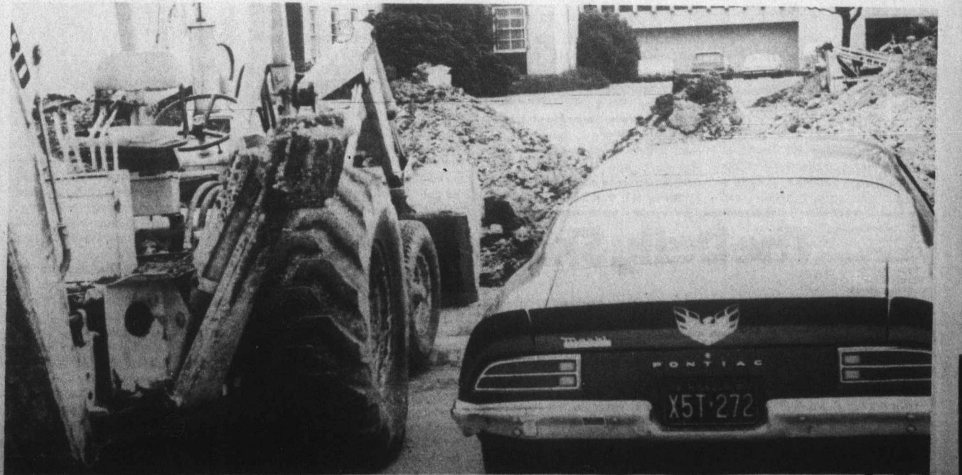
BEAUTY AND THE BEAST—Renewed construction outside of Dan Rogers Hall after several weeks of bad weather made for strange contrasts. One Firebird
