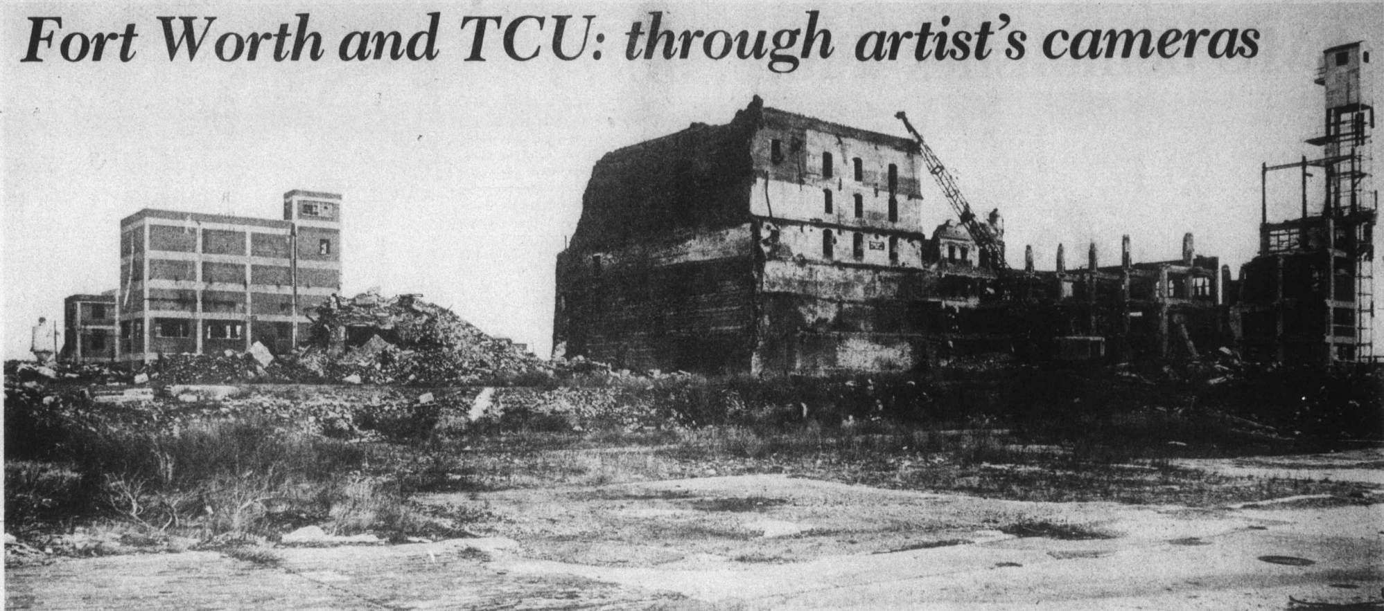
North Fort Worth tells a story of its own. Roger Welder recently photographed this side of the Fort Worth story, where structures are being demolished to make way for the new.
