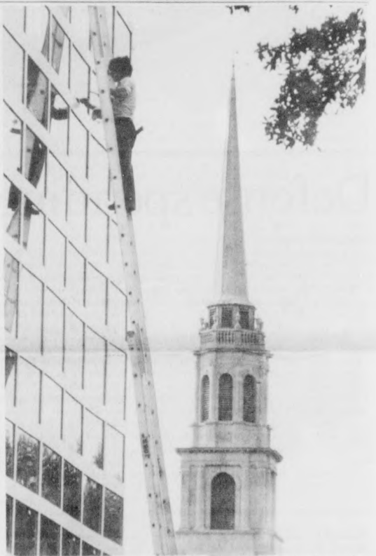
FEELIN' HIGH—A workman puts finishing touches on the glasswork in the new Moudy building. Photo by Ben Neoy
