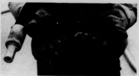
FACE LIFT FOR TENNIS COURTS—Mark Kopp works tediously removing the surface of the Mary Potishman Lard Tennis Center. Kopp sandblasts the old paint without scratching the underlying layer of concrete.
