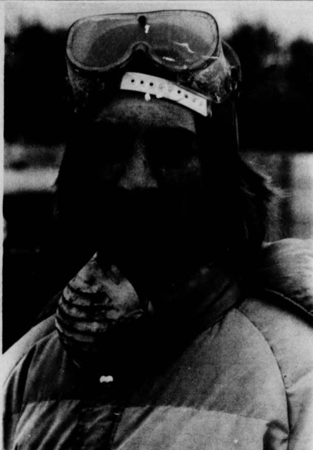
The sandblasting work, contracted by the Bob Edwards Co., began in mid-December and is expected to be completed today. The job was delayed due to the bad weather earlier this month.
