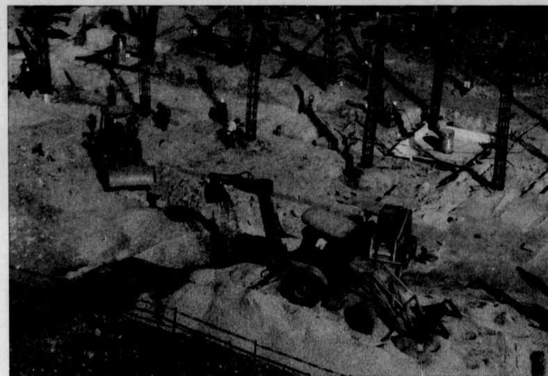
Photo by Sarah Kirschberg/PHOTO EDITOR Work continues on the William E. and Jean Jones Tucker Technology Center as seen from the angle of a camera set on the roof of the Sid W. Richardson Building.
