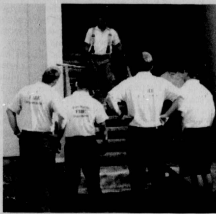
Fort Worth firefighters return to assess damages Monday to the Stonegate Villas after a three-alarm fire.
