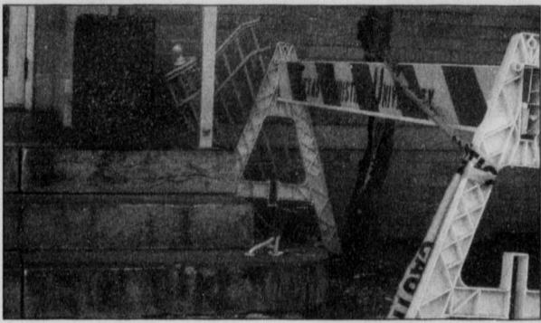
The east entrance of Milton Daniel Hall was vandalized two weeks ago. The concrete stairs were partially ripped out of the ground along with the railing. Two windows of the building were also broken.
