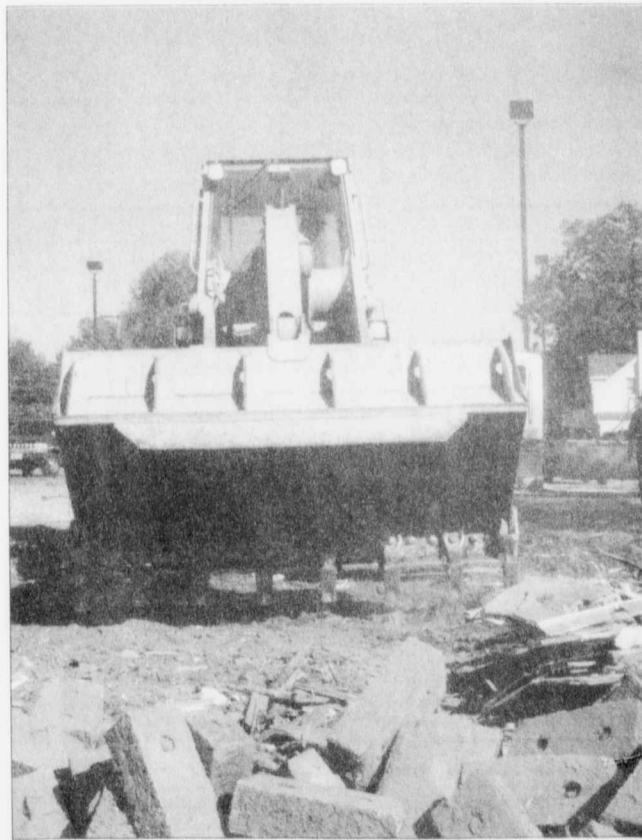
Waddell Excavating destroys the building that once housed the Facility Services office next to the Pastoral Care office on West Lowden to make space for parking across from the Steve and Sarah Smith Entrepreneurial Hall.
