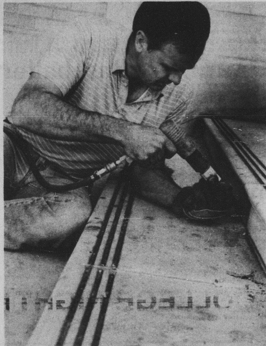
Step in the right direction - Jerry Miller prepares to re-seal joints between steps at Sadler Hall Tuesday. Miller and his partner Jim Laux have been working on the steps all week and expect to be done by March 3. Water accumulation under the steps can cause them to buckle.
