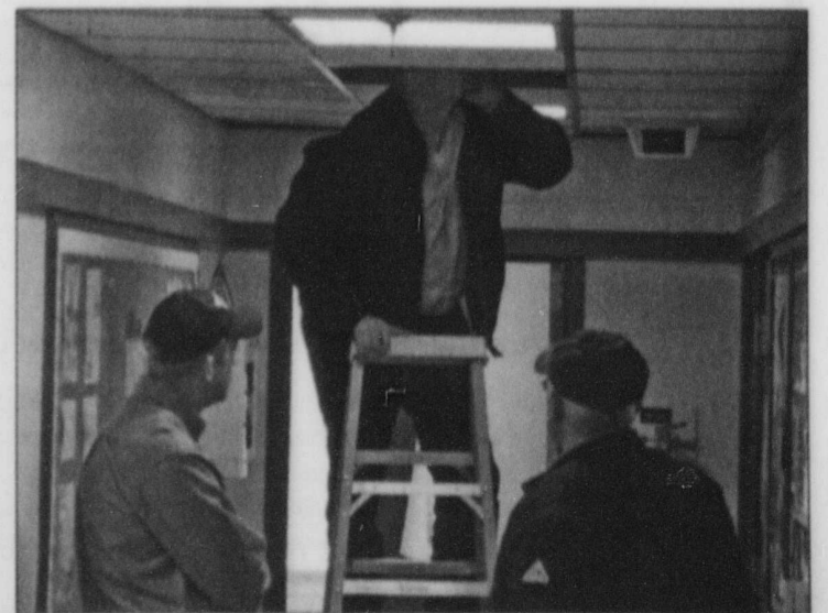
The TCU Physical Plant inspects the air ducts, suspected to be the cause of smoke in the tennis pro shop.
