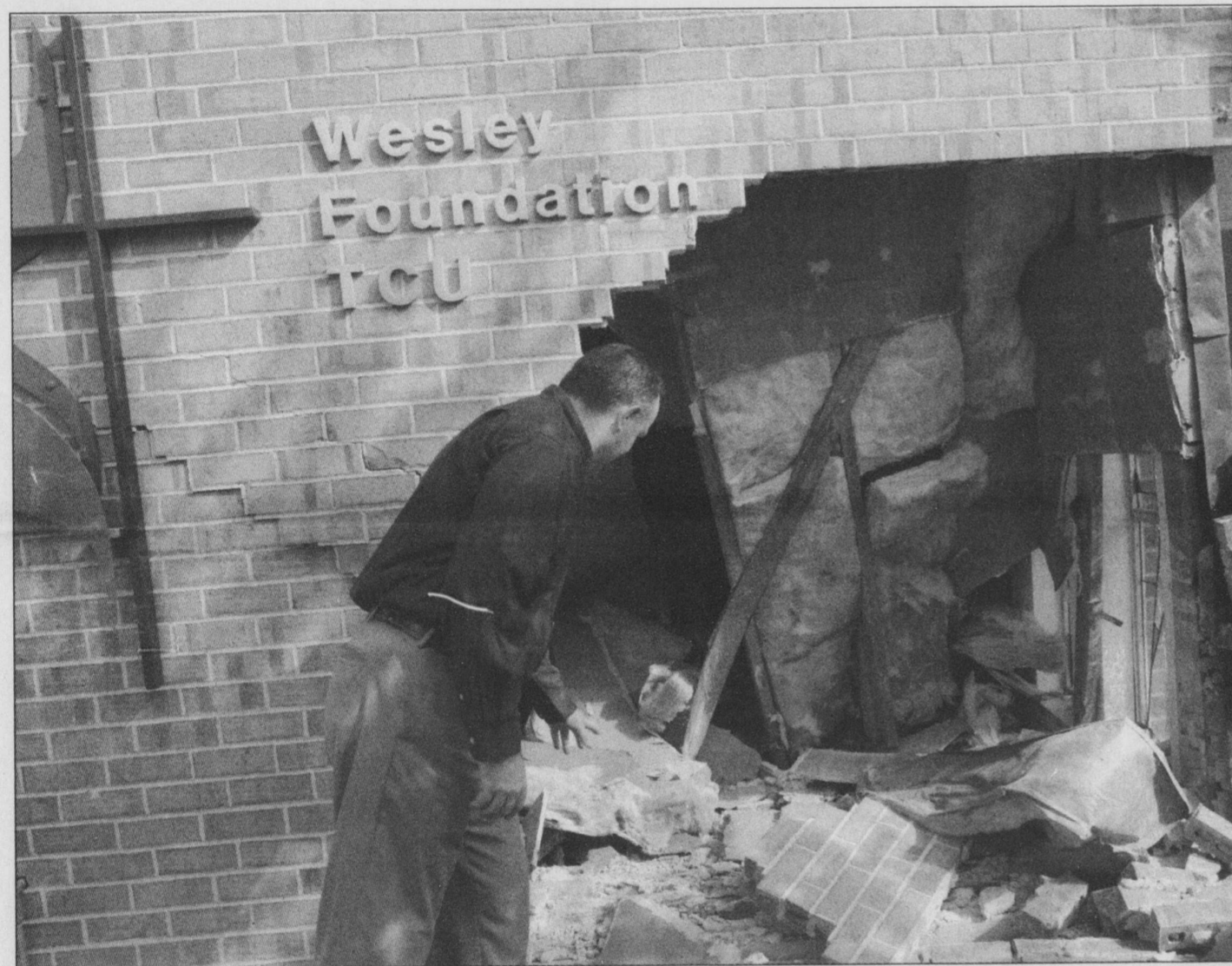
The Rev. Lindsay D. Churchman, United Methodist Church campus minister, assesses the damage done early Wednesday morning by a Toyota Tundra. Between 3 a.m. and 8 a.m. Wednesday, according to the Fort Worth Police Department, a truck drove into the side of the chapel of the Wesley Foundation on West Lowden Street and the license plate of the driver was found at the scene. The Fort Worth Police Department is still attempting to contact the suspect and determine the cause of the accident.
