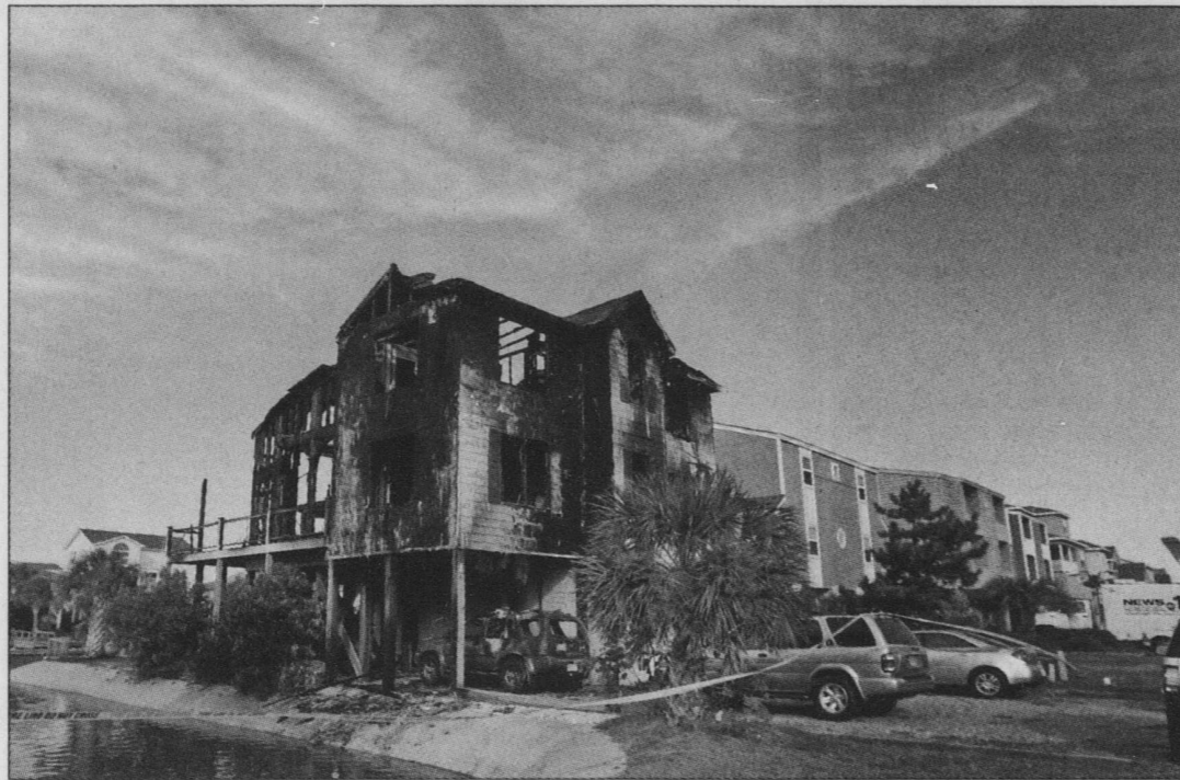
The burned remains of a home are seen Monday in Ocean Isle Beach, N.C. Seven were found dead after the fire, which officials say may have started on an outdoor deck.
