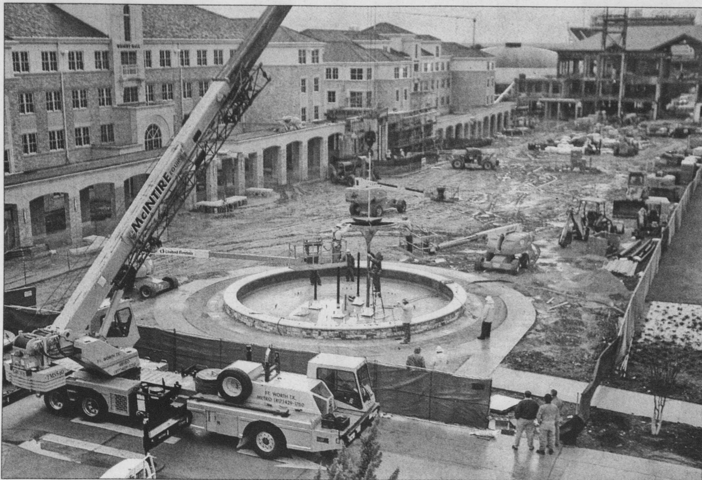
Workers assemble the refinished Frog Fountain on Dec. 12. Jef Larremore, the Web services coordinator for Student Affairs, watched the fountain go up last month and took this photo from the roof of the Brown-Lupton Student Center. To see more photos, visit the Skiff's newsroom blog at blogs.tcuailykskiff.com . If you have photos for the Skiff you can send them to yourtcu@dailykskiff.com .
