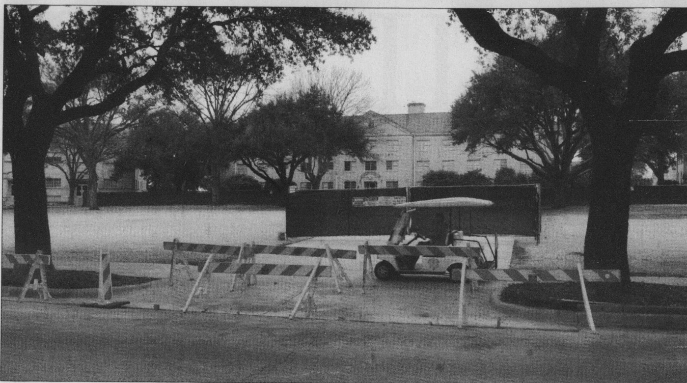
A golf cart drives across the new sidewalk that cuts through Clark Lawn. Friday afternoons on the lawn were spent with students playing sports outside, but the recent construction has put an end to the games and other activities. For the story, see page 5.
