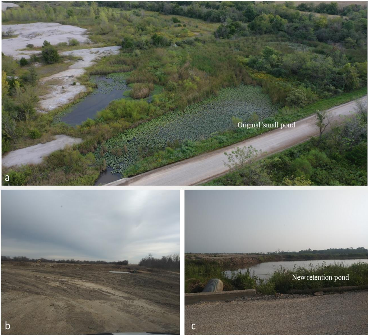
Figure 4: a) Pre-construction – September 2019, b) during construction – January 2021, and post construction – July 2021 images of earthen dam and new retention pond. Before image courtesy of Quapaw Nation Environmental Office.
