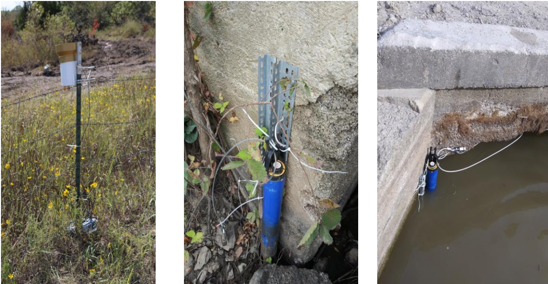
Figure 6: Rain Gauge, north location equipment and south location equipment installations, respectively.
