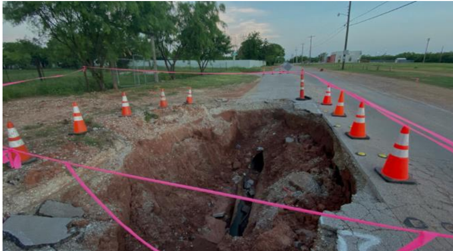
Figure 9: A recent (2021) sinkhole that occurred in northern part of Abilene caused significant property damage (Henderson, 2021)
