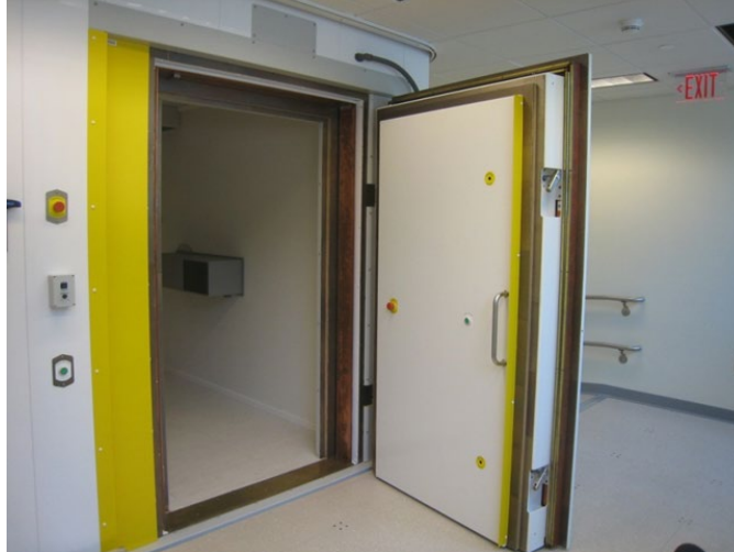
Figure 4: Magnetically Shielded Room where the MEG is located. The patient is inside the room accompanied by his/her caregiver while the rest of the personnel are located outside. The room is equipped with an intercom system to ensure the patients safety, along with audio-visual components and adjustable lighting 24 .
