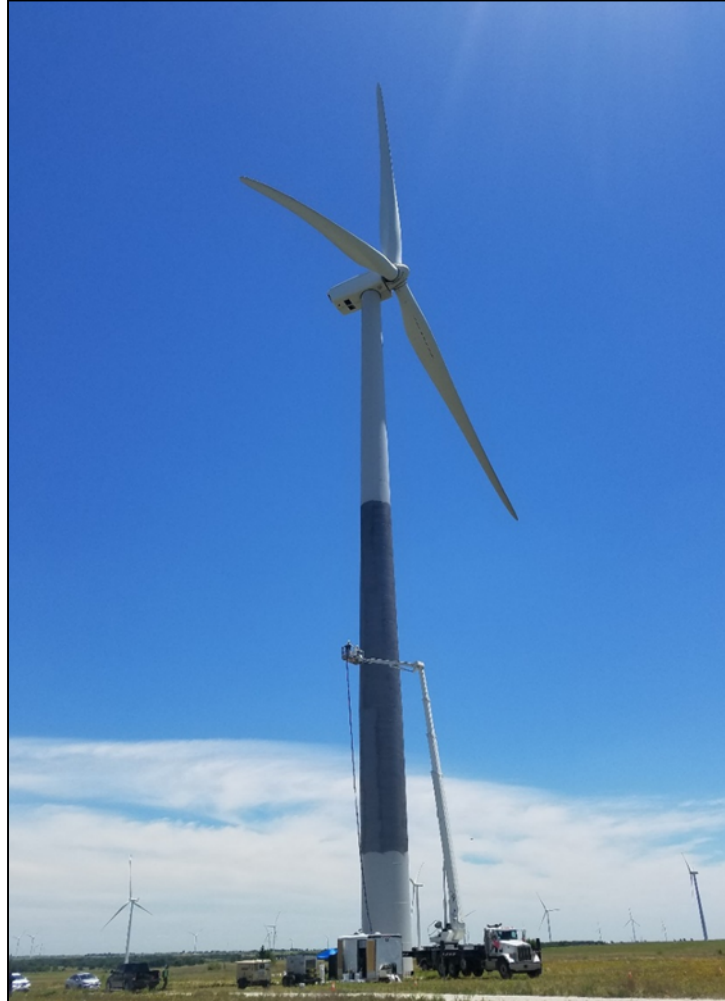
Figure 7: Texture coating application at a wind turbine at Wolf Ridge in June 2017.
