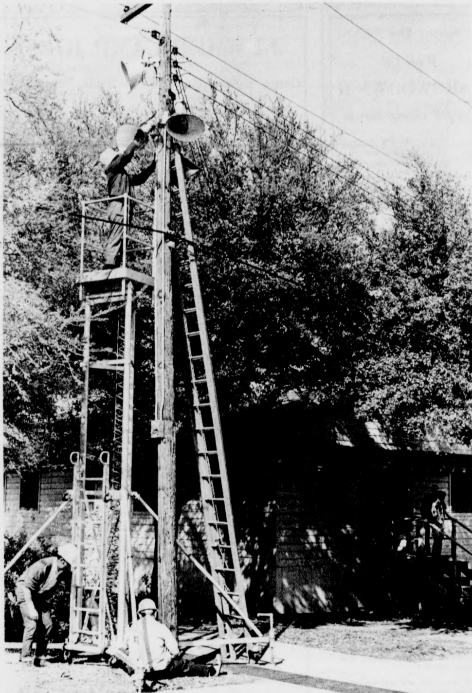
LIGHT WORK —Maintenance men carried out simple repair work this week on a cluster of lights near the Security Office. Using a hydraulic lift, workmen replaced several lightbulbs. The work did
