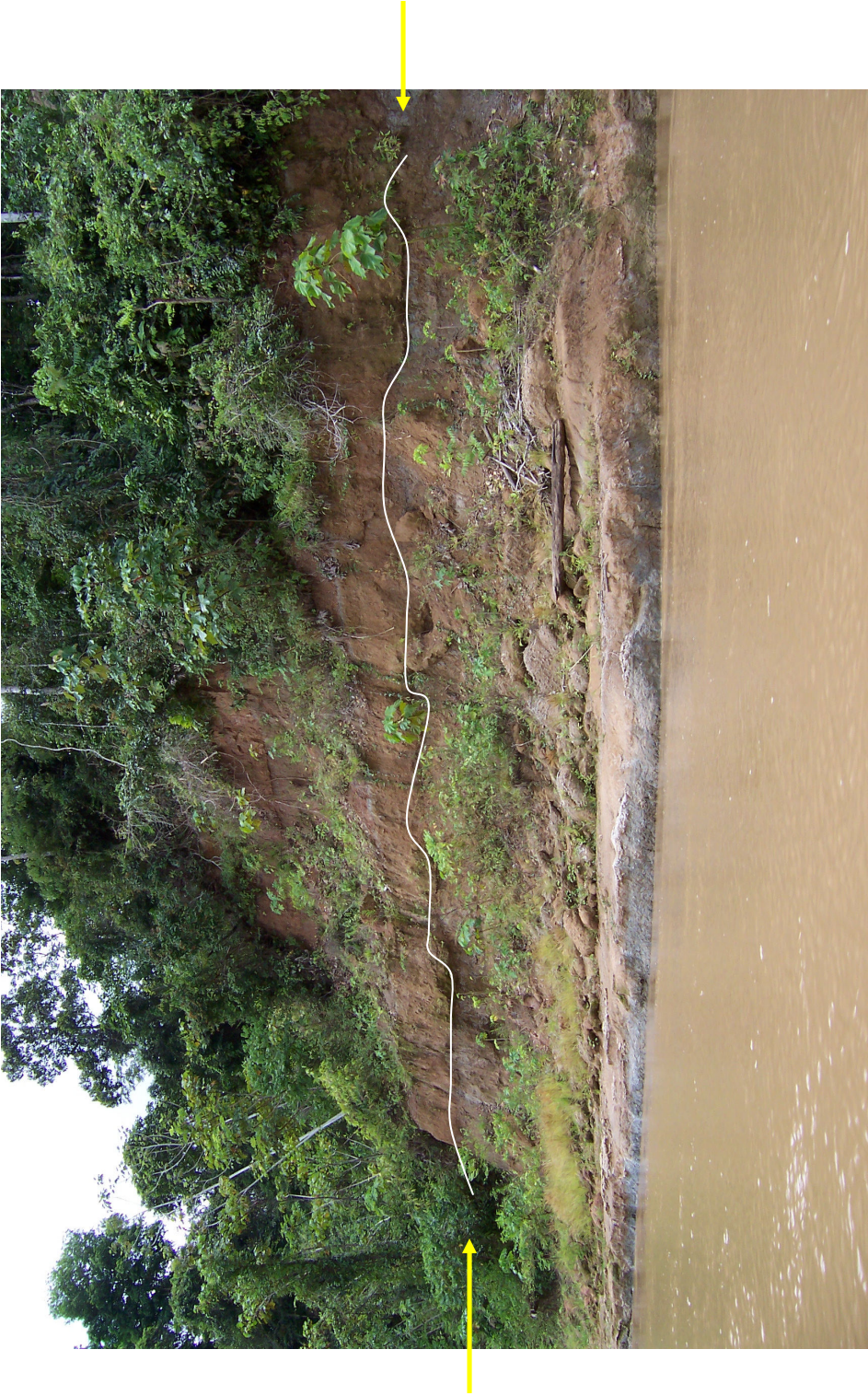
Fig 2.6.2: Erosion at a river bank. Many river banks in the study area are unstable. Note the shallow rooting depth. The breaks (shown in white line) running along the soil profile suggest historical soil deposition. The breaks may be attenuated by wet/dry cycling of soils.
