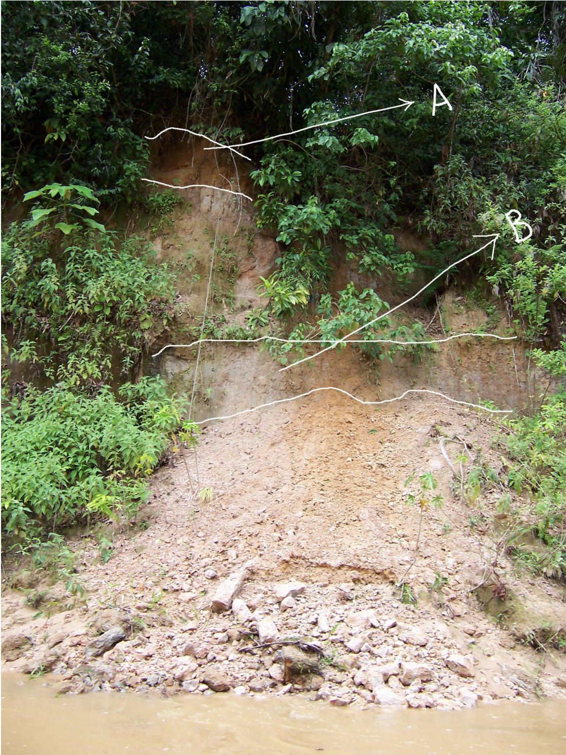
Fig. 2.6.8: Riverside failure. This is a small translational slide. Note the second order failure from the upper scarp. The lower scarp (B) is the older one with dark colored organic lining on the surface. The upper scarp (A) is fresh.
