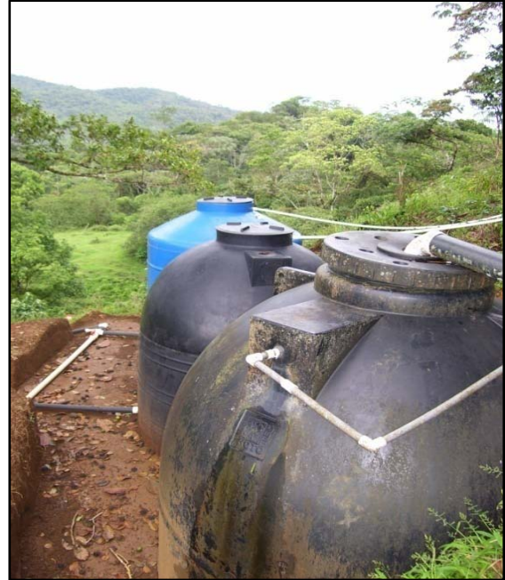
Figure 6: Two holding cisterns send water to the houses by force of gravity. The other cistern sends water to the tank in figure 5.
