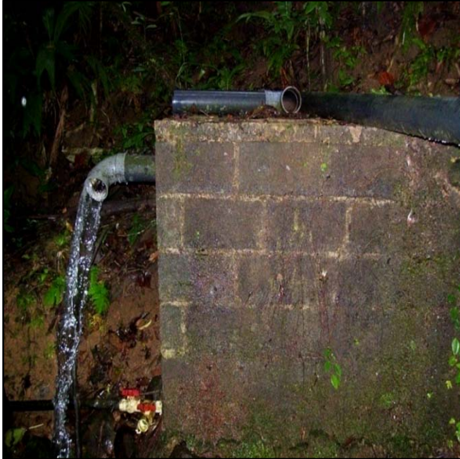
Figure 5: Circulation tank allows constant movement of water when all supply tanks are full. A similar structure exists at the research station water source.
