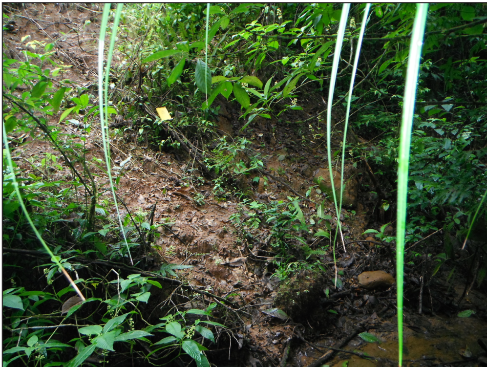
Figure 11. Riparian slope failure located between reaches A and B. Top – Slump scarp. Bottom – Slump toe intersecting the channel margins. Field book for scale.
