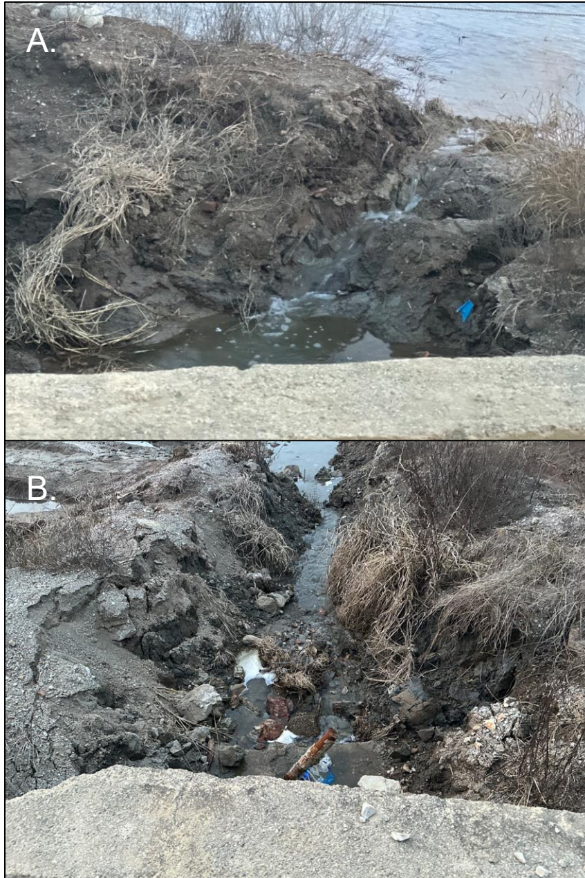
Figure 17: Downcutting of the stream channel upstream (A.) and downstream (B.) of the Bird Dog South Culvert.
